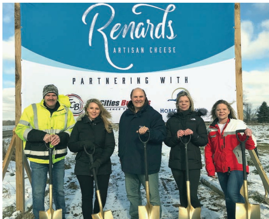
Renard's Cheese broke ground last week on an expansion that will ultimately take the plant from 3 million pounds of cheese to 12 million. In the above photo are: Mike Pribek, plant manager; Ann Renard, president; Chris Renard, vice president; Jean Chase, human resource director; and Joni Nessinger, production manager at Renard's Cheese during groundbreaking events.
